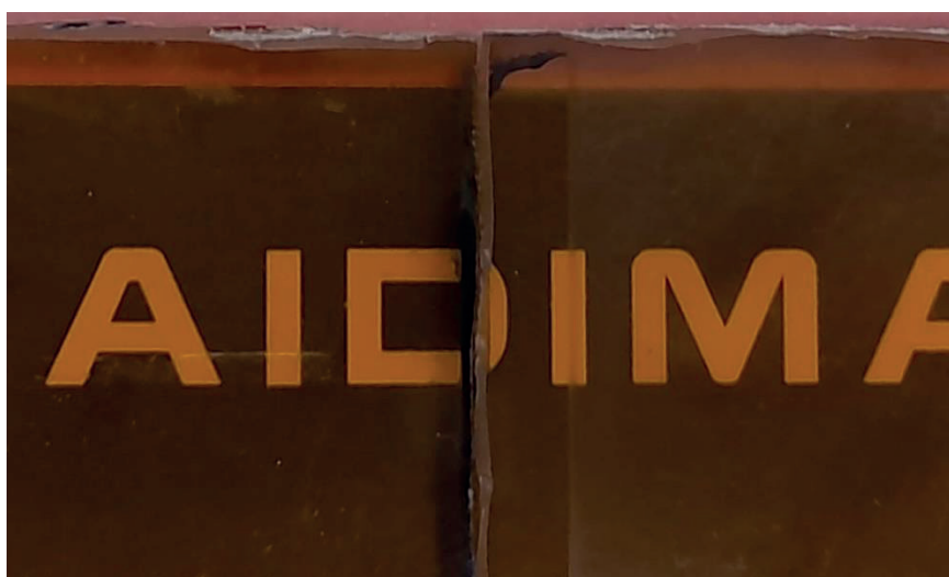
Image 15. Detail of matting surface because of weathering.
